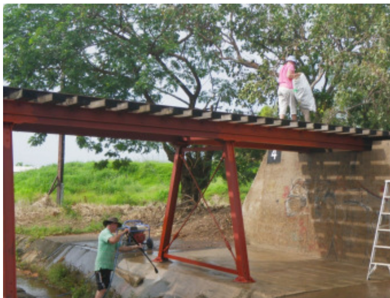
Below the bridge: Kerry Moran water blasting Above the bridge: Di Lunn on emu parade
